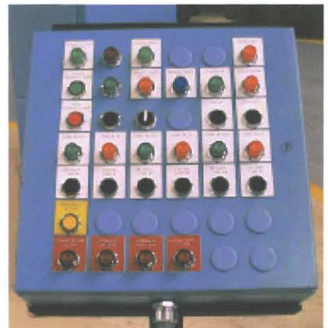
Trim Press Operator Interface
